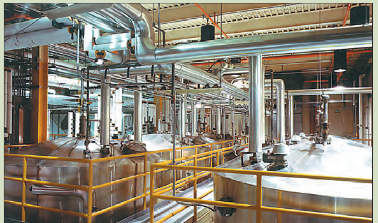
Danisco, Olathe, Kansas - Austin completed a major plant expansion for this facility that produces food additives used in a wide variety of dairy, meat, confectionery, beverage and bakery products. The expansion provided for service to North American market with products previously imported from Denmark.
