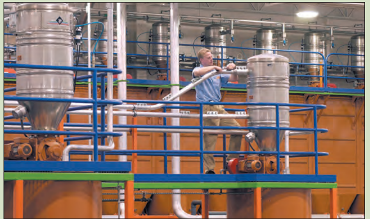
Mother Parkers Tea & Coffee Inc., Fort Worth, Texas - Austin provided site-location, design, engineering and construction services for this new coffee roasting and distribution facility for Canada's largest coffee supplier. The plant was designed to produce 20 million pounds of coffee per year, with flexibility to produce four times that in the future.
