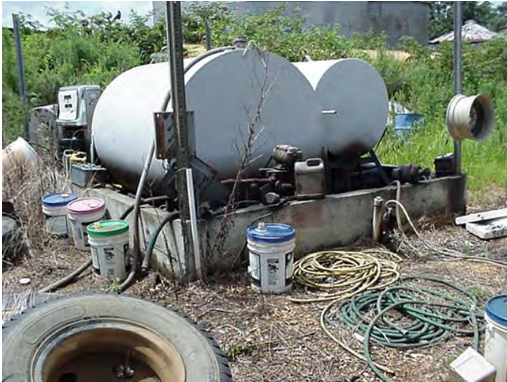
Parcel #24 - N 36° 53' 58.4", W 88° 39' 35.1" - Fuel Oil Tanks in Diked Area
