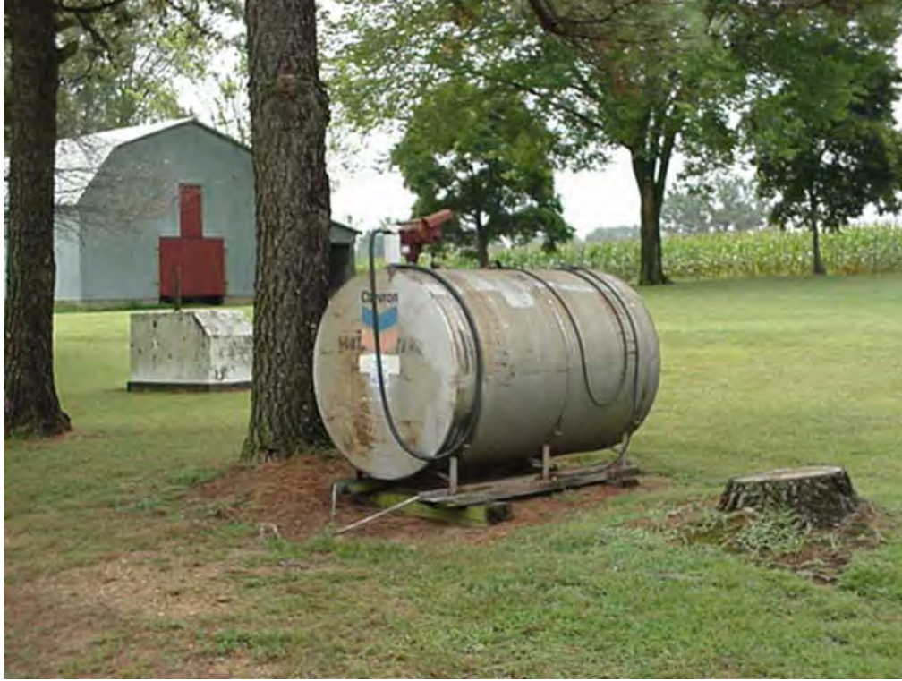
Parcel #41 – N 36° 53' 28.4", W 88° 39' 50.0" – Above Ground Diesel Fuel Storage Tank
