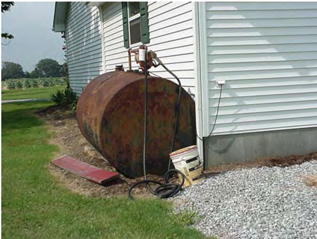
Parcel #54 – N 36° 53' 36.2", W 88° 40' 14.4" – Above Ground Diesel Fuel Storage Tank
