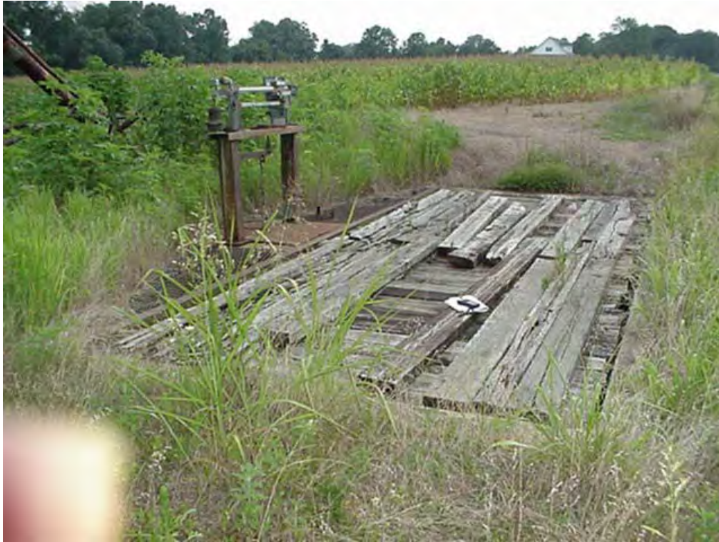
Parcel #55 - N 36° 53' 37.2", W 88° 40' 03.4" - Weigh Station Above Grated Pit
