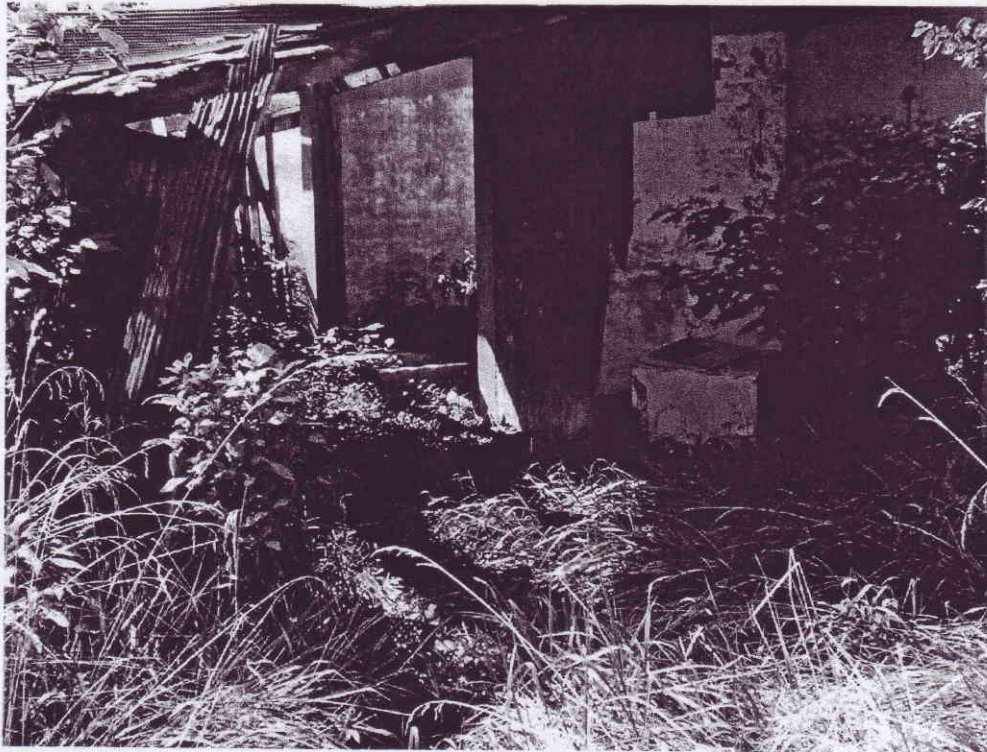
Figure 16.3.9. Building formerly used as swine pen. It consists of an addition to existing shell loading plant structure.
