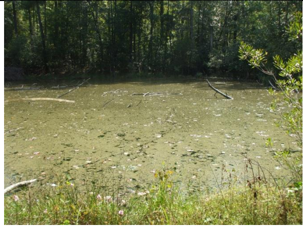
PHOTO 33 – The concrete-lined cistern has not been in use for a number of decades
