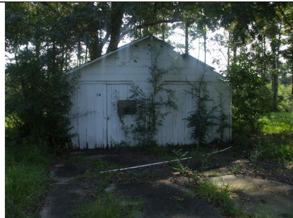
PHOTO 45 – SUPERINTENDENT'S HOME garage in rear of home. This structure appears to have asbestos siding.
