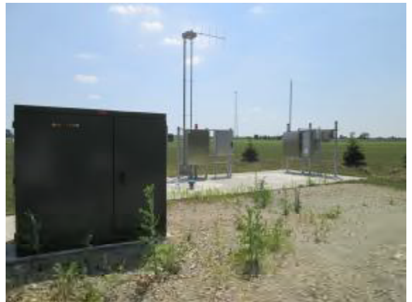
Photo #4: Viewing the small lift station.
