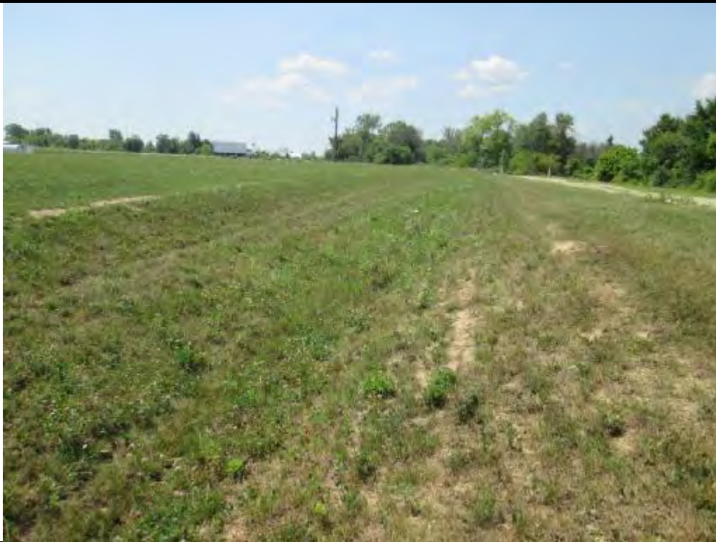
Photograph # 5 Description: Drainage Feature #5 located on the southwest portion of the Site. Project # 16IN0383 Project Name: Wabash Industrial Park Date: 7/20/2016
