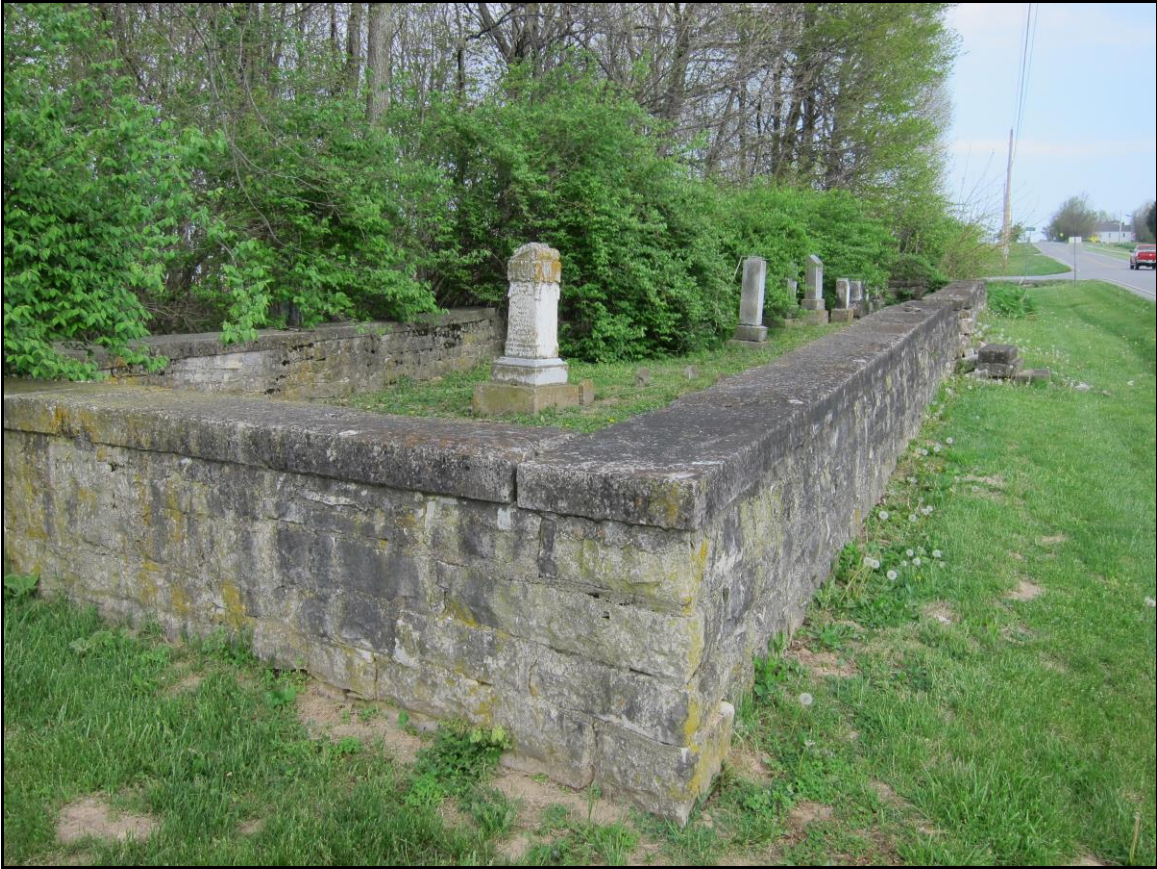
Photo 9: View, facing north along the west side of SR 771, of a walled section at the northern edge of AL 3 (OGS 5194)
